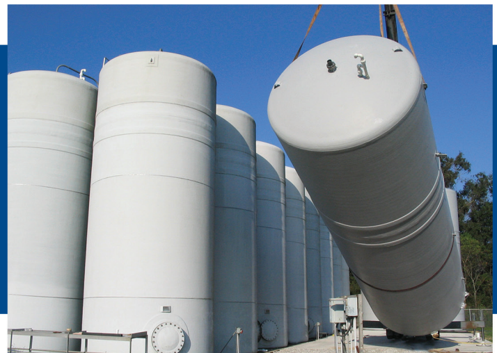
30,000 gallon food grade liquid storage tanks, 12' diameter x 36' sidewall height.
