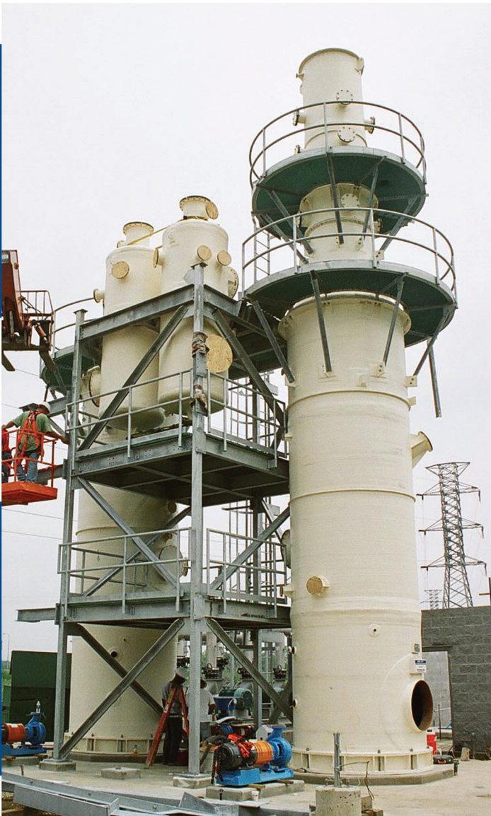
Sulfur recovery from biogas via liquid scrubbing, included 12' diameter x 36' sidewall, skirt supported cone bottom oxidizers, 3' diameter x 13' SSH x 14' absorber vessel and two 3' diameter x 11' SSH, dish bottom knock out pots.
