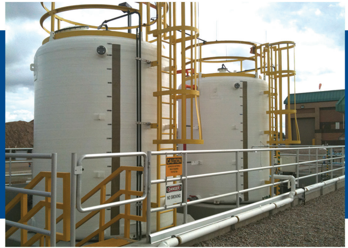
7,000 gallon Sodium Chlorite tanks for water treatment, 10' diameter x 12' sidewall. Furnished complete with FRP ladders and handrails.
